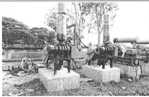
Pumps provided to Aeration Tank
